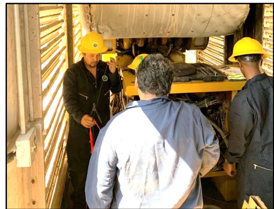
BEL team connecting the generation unit to the Caye Caulker power system.
